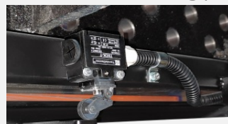
limit switch - crushing protection
